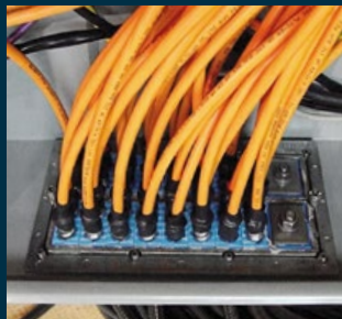
Electric heat trace cabinets
