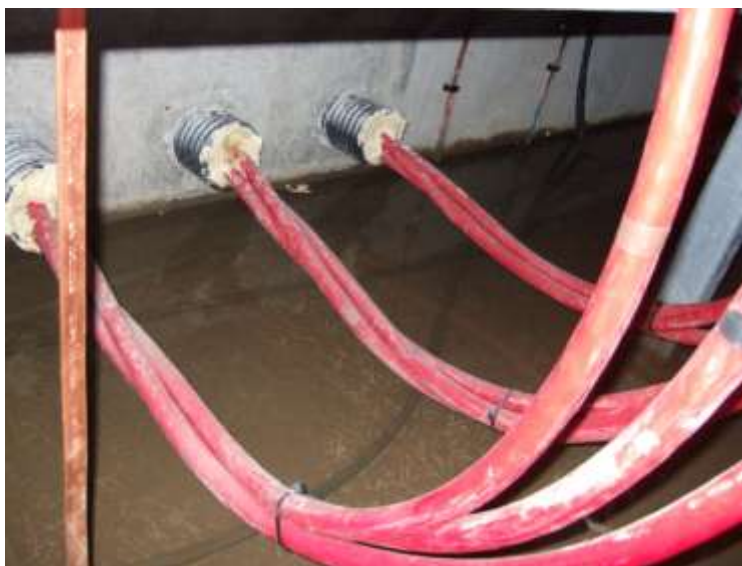
Figure 3 – Flooded cable trench
